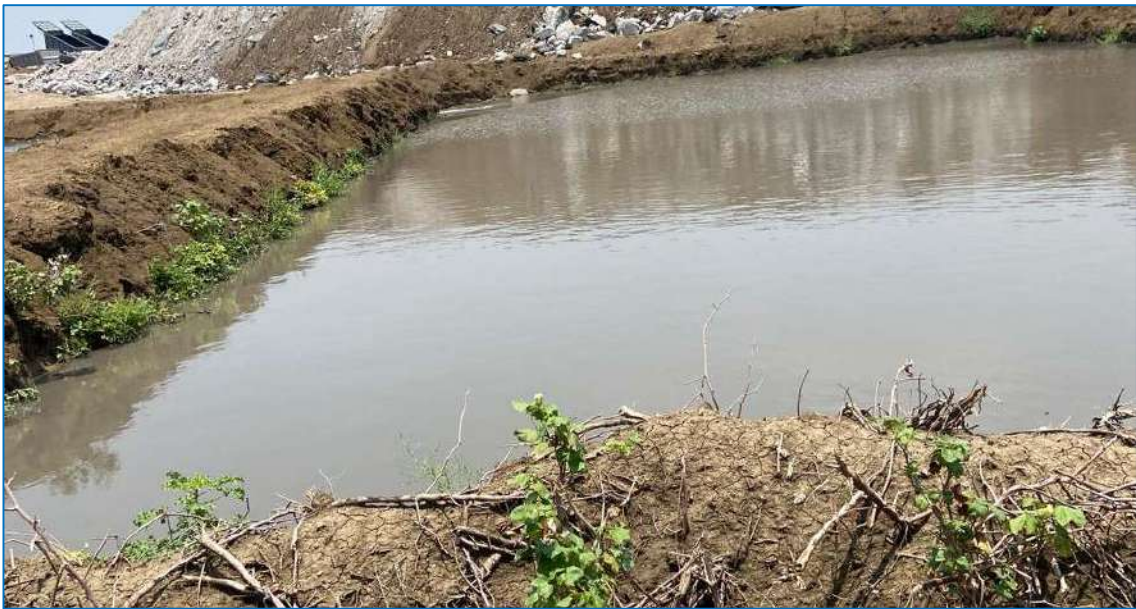
Series of Sedimentation tanks (3 no's)
