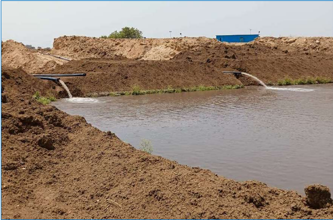
Mine seepage water pumping into sedimentation tanks
