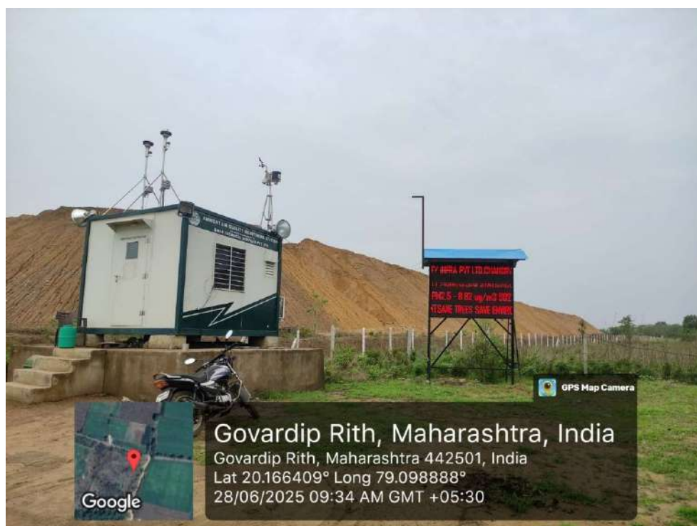
1. CAAQMS under operation
