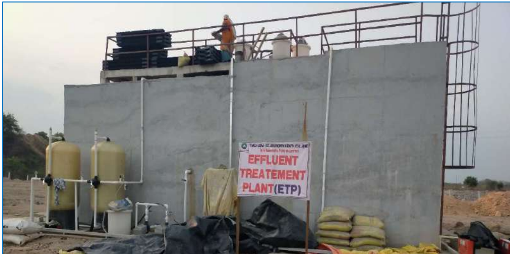
ETP of 100 KLD ready for operation
