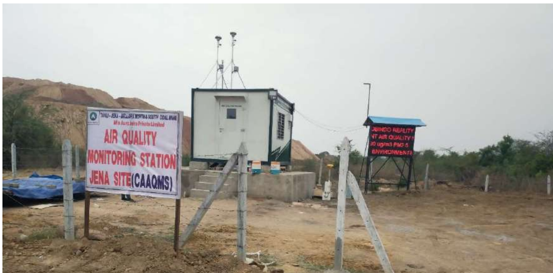
1. CAAQMS under operation
