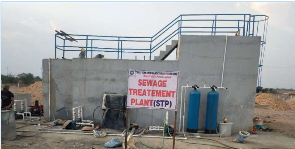
STP of 44 KLD ready for operation
